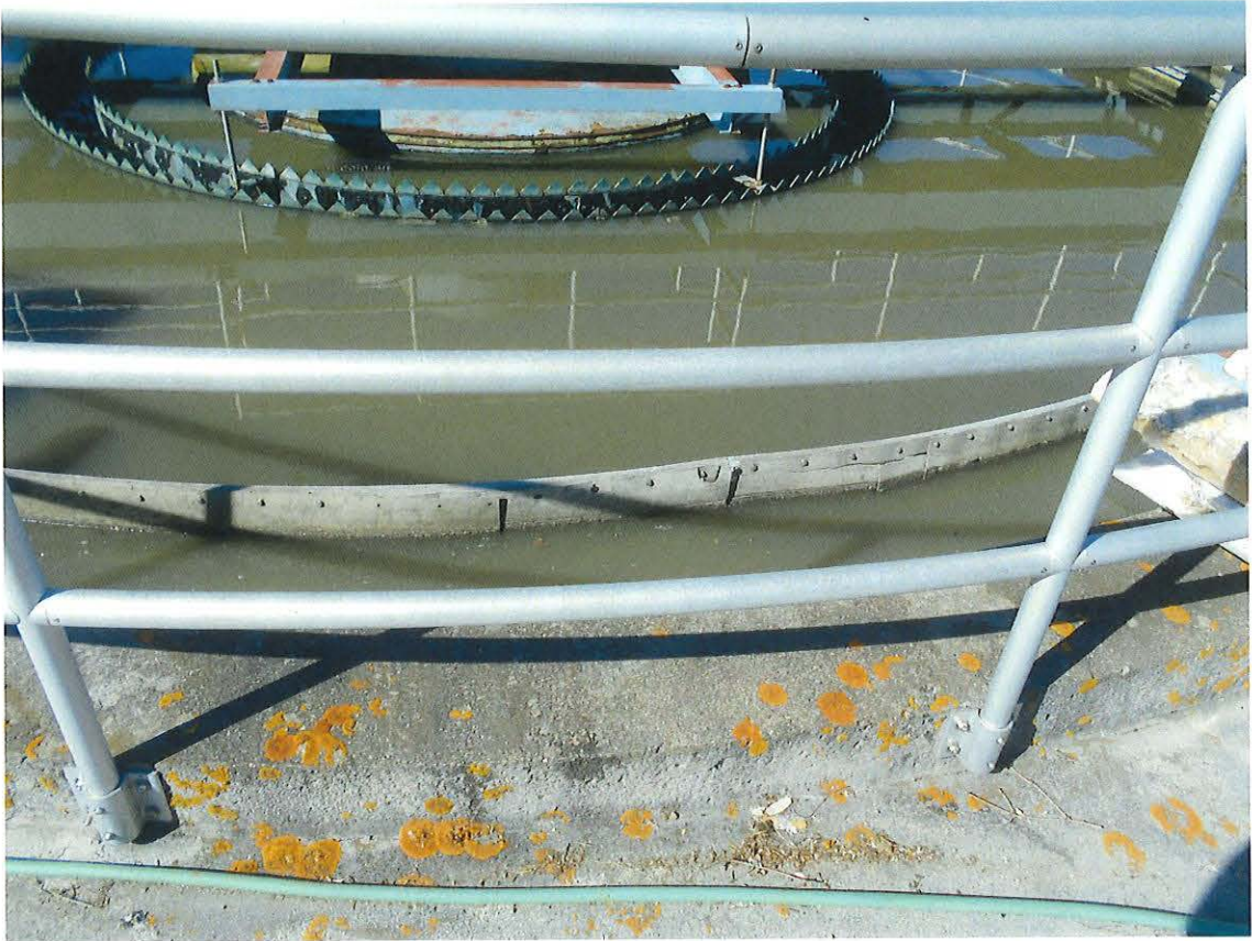
Failing Imhoff tank
