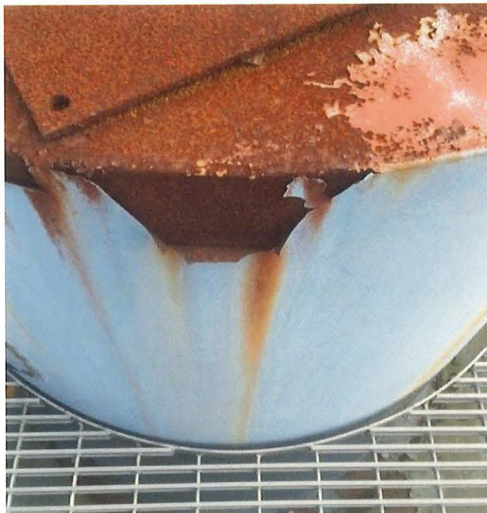
Corroded Imhoff Tank
