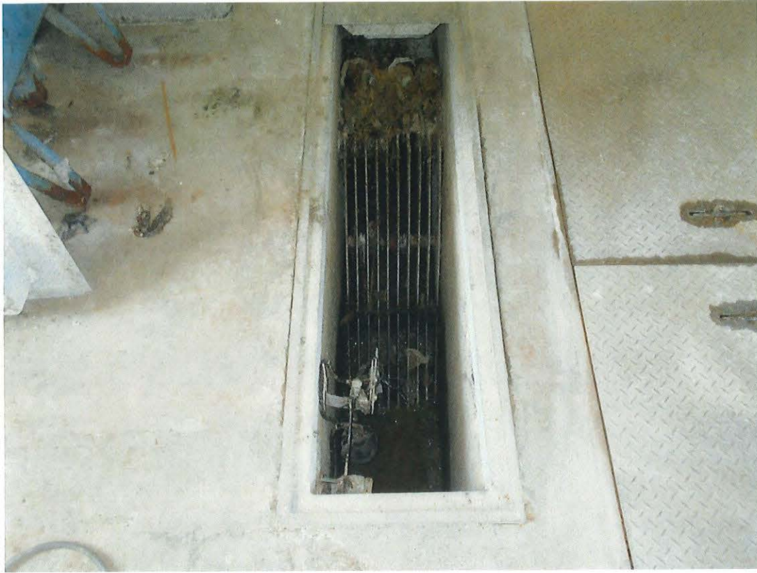
Existing Manual Bar Screen
