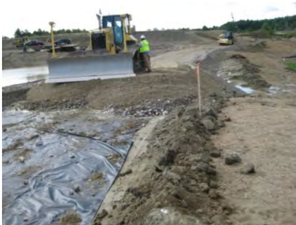
A woven geotextile fabric will strengthen a road constructed over soft or poorly drained soils.
