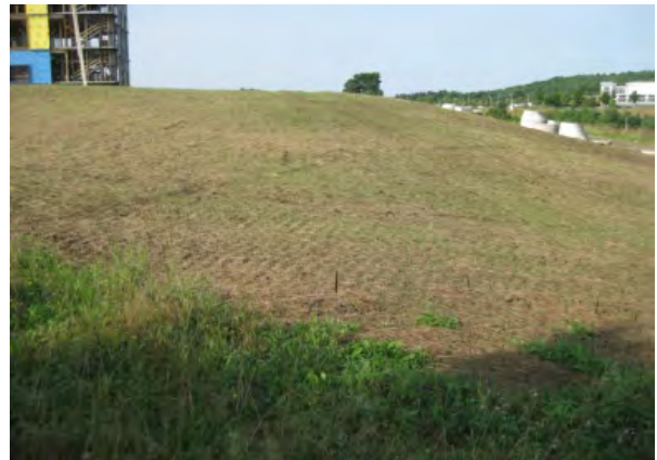
Inspect periodically the revegetated area. To be considered stabilized, 90% of the soil surface should be vegetated or the area may need reseeding and mulching.
