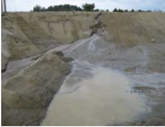
Seeping slopes are found at cuts that intercept the groundwater table. Often, riprap over a layer of drainage gravel is the only appropriate stabilization measure.
