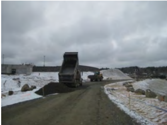
The preferred road construction is above natural ground elevation for positive drainage. Cuts and fills are more of the norm for roads constructed along the contour of sloping sites.
